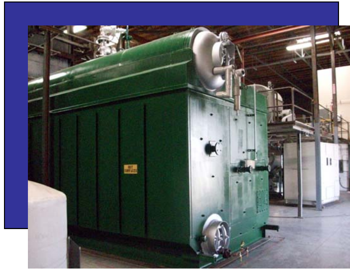
The Recycled Steam Boiler is prepared to make over 30,000 pounds of steam an hour to power the electricity generating turbine.
